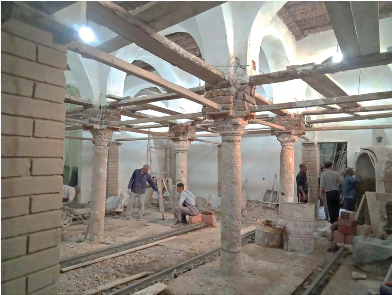
Fig. 4 - Interior of the prayer room with Roman columns and wooden tie rod system (source: photo by the authors, 2020).
