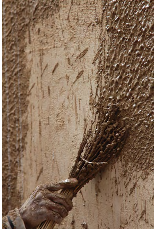
Fig. 9 - Application of the plaster using a palm branch (source: photo by the authors, 2020).
