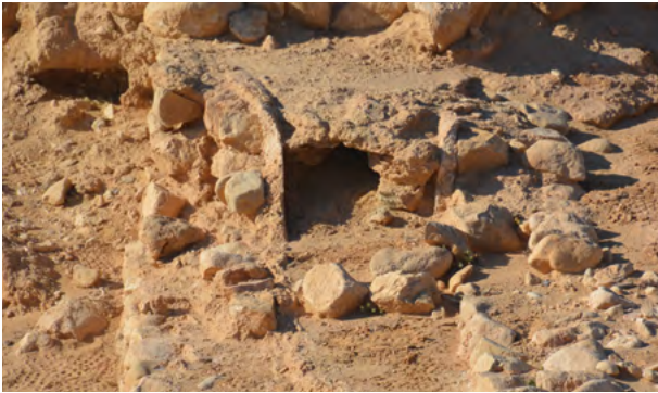
Fig. 4 - The channel in a position close to the CW Sidi Khellil provincial road. To be noted the mortar spread in such a way as to cover the upper part of the sidewalls of the duct /photo by the author).
